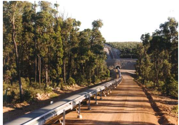
Figure 1. Low Profile Ground Based Conveyor – Australia Muja Overland Conveyor
